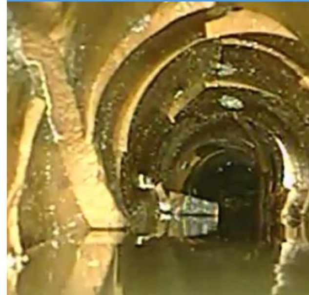
Clay Sewer Pipe Failure
